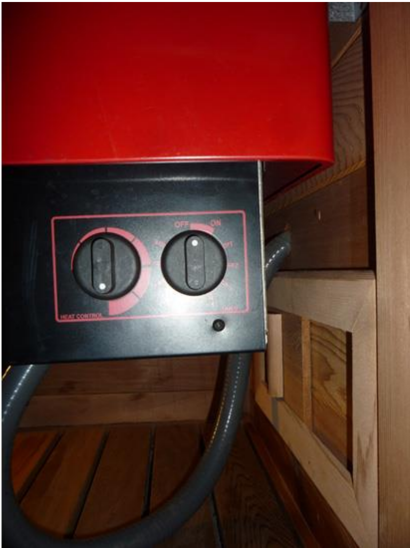
Wall mount heater, vent and conduit
